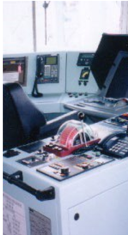
Propulsion Control System
