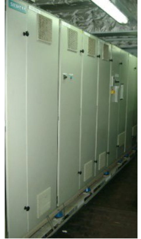
AC Variable Speed Drive
